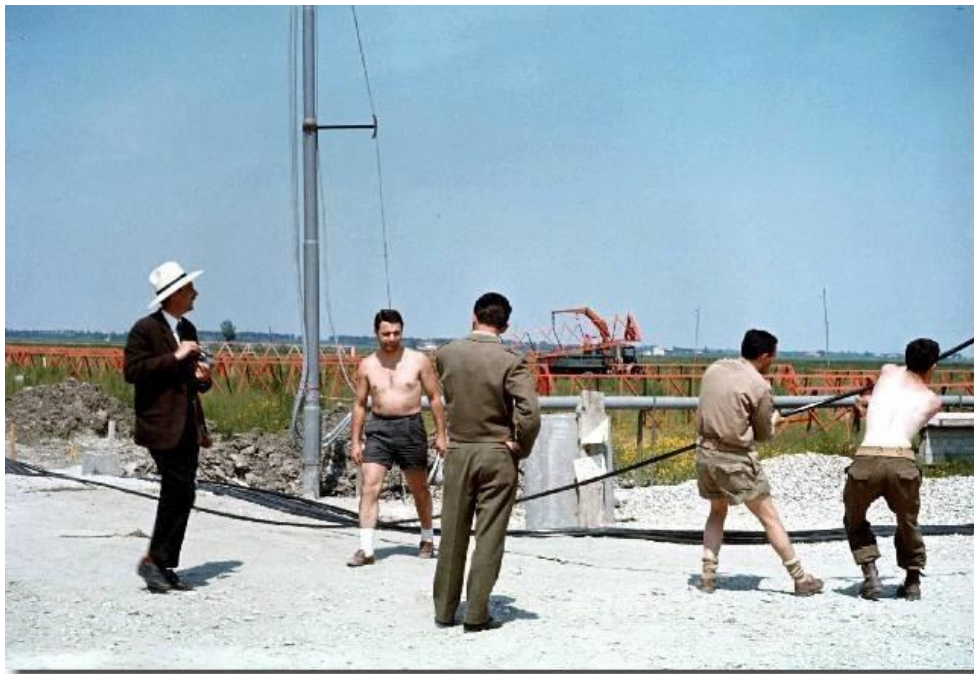
The military corps of engineers involved in laying coaxial cables in 1964. Marcello Ceccarelli and Luciano Baldeschi can be recognized on the left. Credits: INAF-IRA
